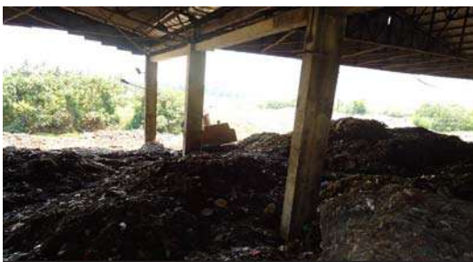
Figure 6 Tilted columns in Brahmapuram
