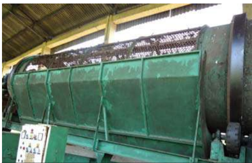
Figure 4 Trommel in Brahmapuram
